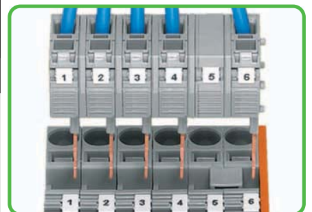
The test plug modules are directly inserted into the jumper contact slots of the current bar (picture shows 284 Series).
